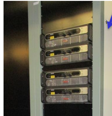
New power supplies for downstream optical matching
