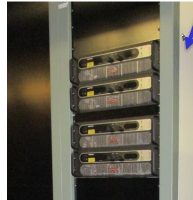
New power supplies for downstream optical matching
